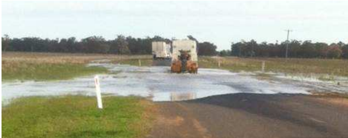
Warren Road Flooding
